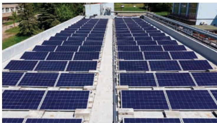
LX CZT solar heat generation facility
